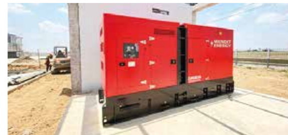
Installations fixes de conteneurs solaires OFF-GRID
